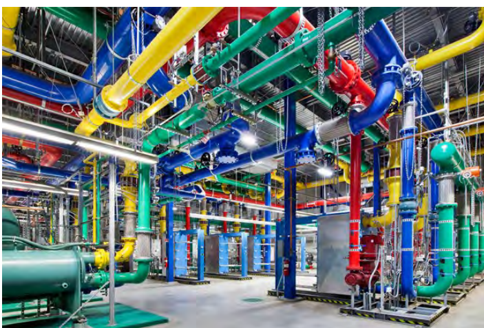
A behind the scenes look at one Google's data warehouse centers. Cables and tubs such as these are just a part of what makes up the information superhighway, as referenced in Andrew Blum's Tubes: A Journey to the Center of the Internet . Photo courtesy of Google Data Centers Photo Gallery 2012
